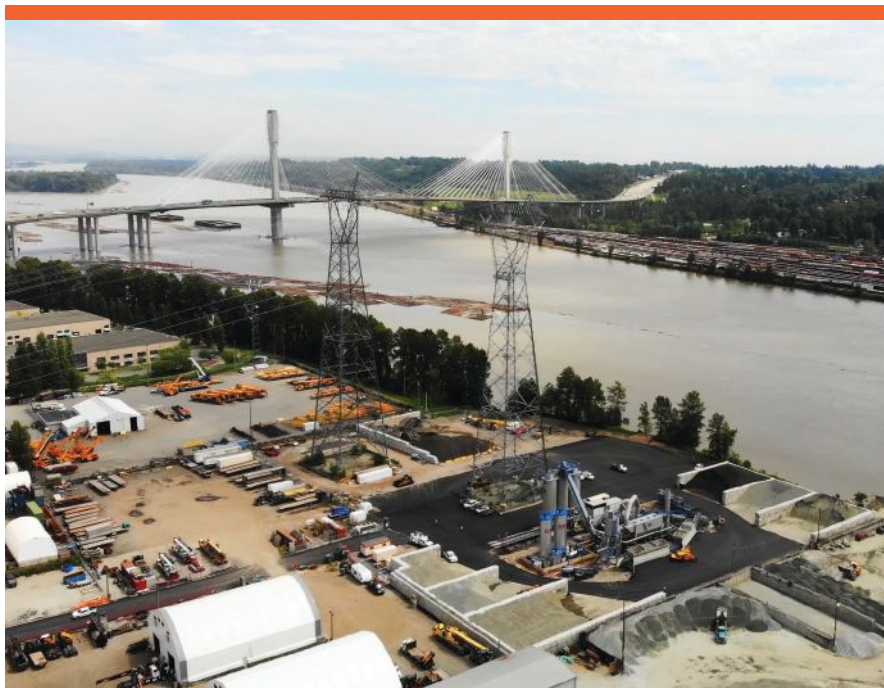
Despite only remote assistance being available during the assembly and commissioning phases of the plant, the project went relatively smoothly. All Roads Construction produced over 100,000 tons of asphalt from its new plant in the first four months.
