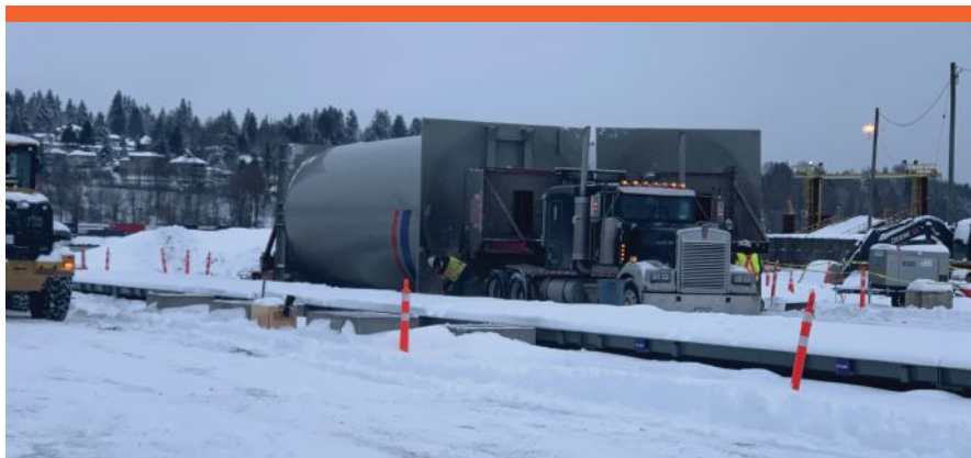
The COVID-19 coronavirus pandemic was declared when All Roads was about one third of the way through construction of the new plant. Photos courtesy of All Roads Construction.
