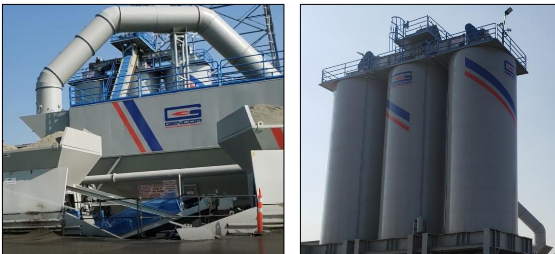
Figure 2: Drum Burner/Dryer System (left) and HMA Silos (right)
